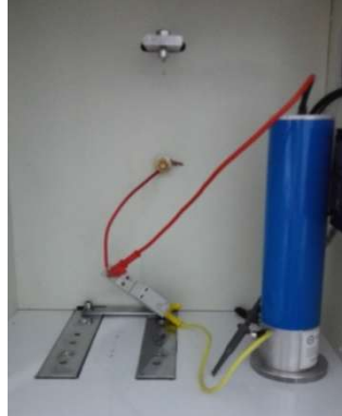
Fig 5 20kV Voltage divider
